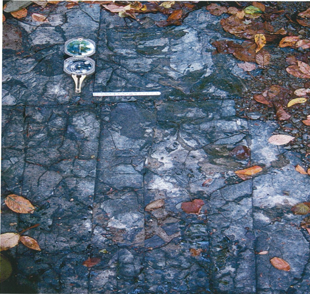
Figure 16: Detailed view of the jointing in Wagener Glen.
