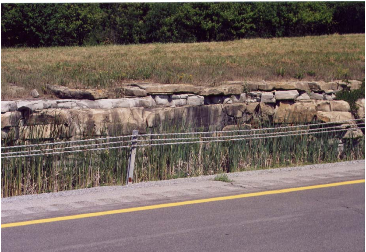
Figure 2-5 Predominantly Buff-Weathering Dolomitic Limestone Beds Typical of the Pamela Formation Sandwiching a Light Gray Weathering Micrite Layer. Location Station BRO-1
